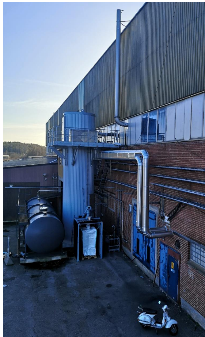
Above: This shows a picture of how the verification of our flue-gas cleaning technology now looks in our plant in Åsensbruk
